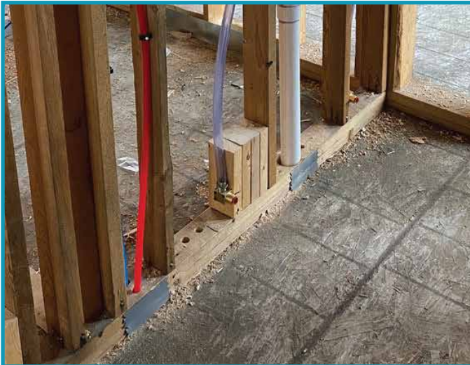
90-degree rough in nozzle installed low on wall to dry across floor.
